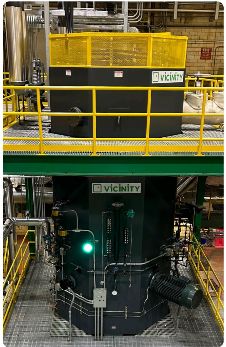
Vicinity's first 42MW electric boiler that was installed at our Cambridge facility.
